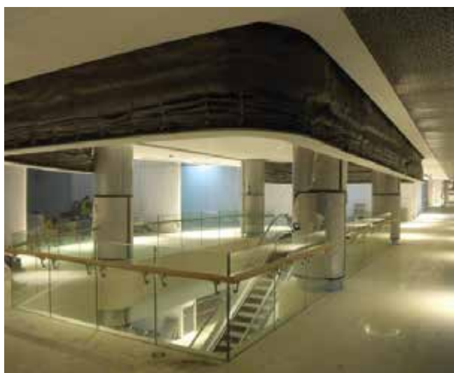
Fire rated fabric shutter at ION Orchard. In the event of a fire, these shutters confine the flames and prevent spreading.
