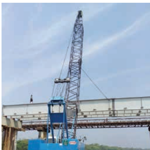
A 55-tonne crawler crane working on a bridge construction project in the Bago Division of Myanmar.
